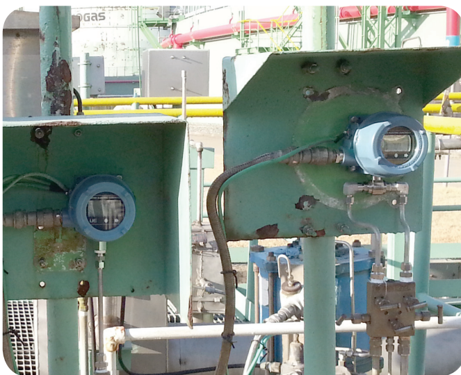
Natural Gas Monitoring
