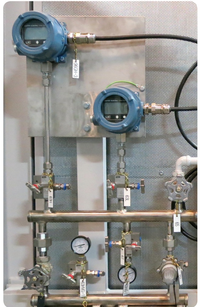
Seal Pressure Monitoring
